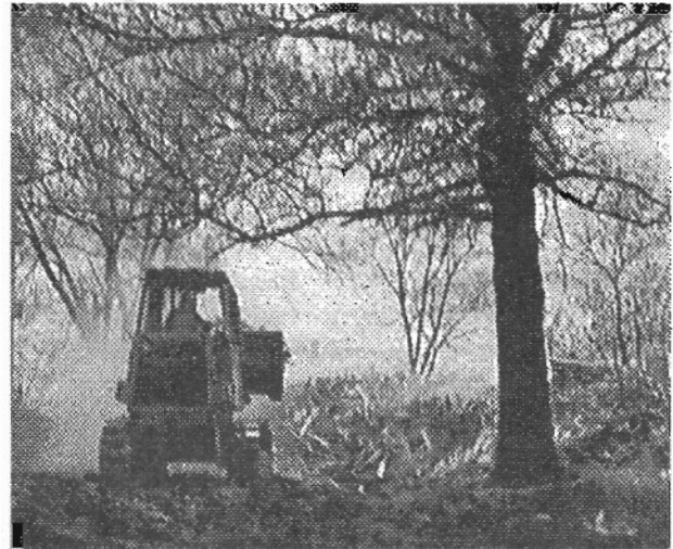
Another piece of Lenexa history was lost to the bulldozer April 20. The Rosner farmstead, a familiar landmark on the corner of 95th and Lackman for years, was destroyed to make way for development.
